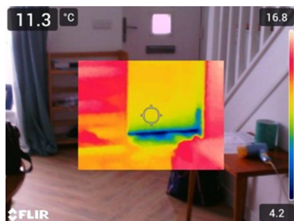
NOWHERE TO HIDE: FLIR thermal imaging shows exactly where the warmth is leaving your house.
